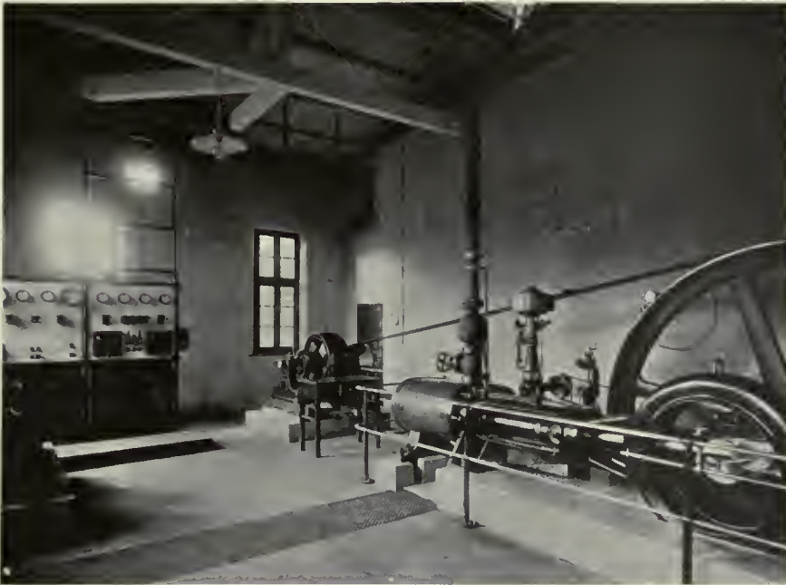
INTERIOR OF THE POWER-STATION AT HANKOW, ERECTED BY THE SIEMENS SCHUCKERTWERKE.
